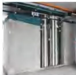
M&E connection to riser
